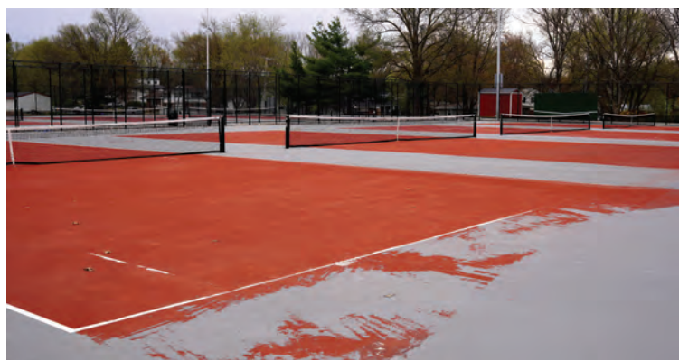
New tennis courts before being repaired for delayed opening. PHOTO BY KATE MEIS
